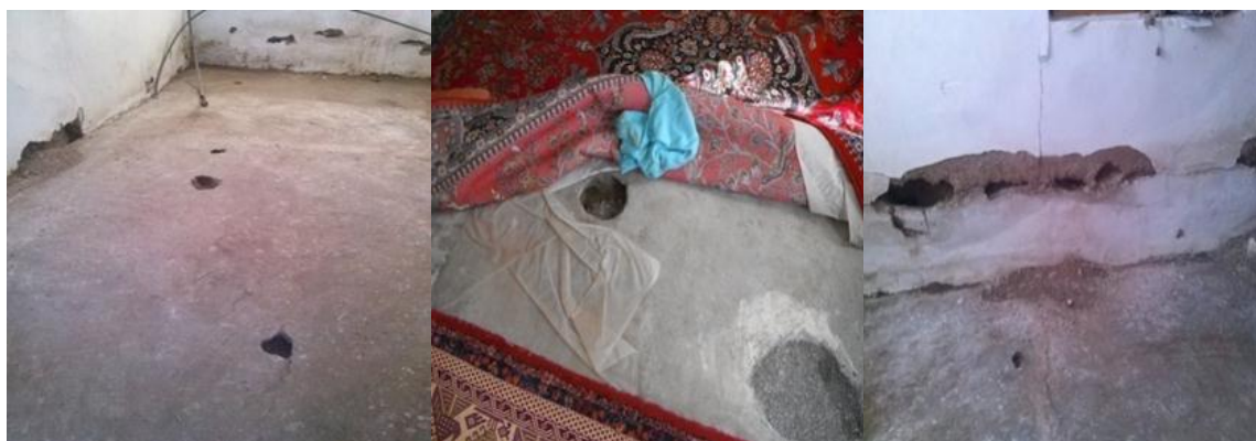
Fig. 2. Effects of rodent infestation to houses in Najaf Abad village; ruined floor of residential houses
